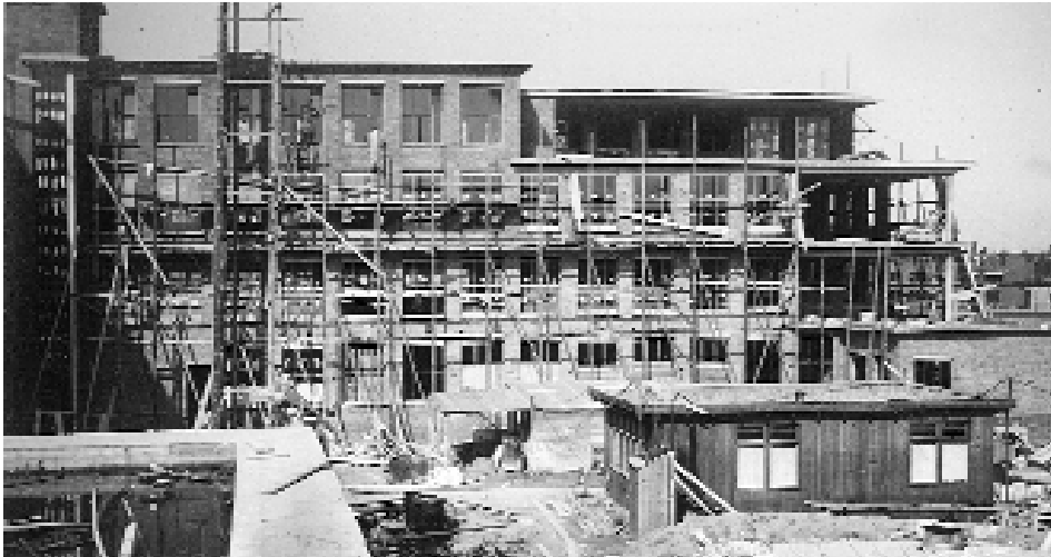
The new Sophia Children's Hospital and Infant Clinic under construction, mid 1935. The wing intended for the Infant Clinic left is largely finished; the Children's Hospital block is still in scaffolding.
